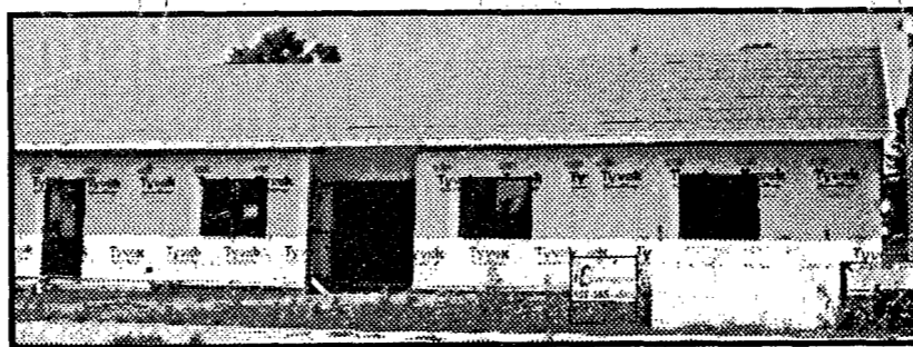
Work on the Lied Winside Public Library is progressing; plans and selections are being made for inside work.
